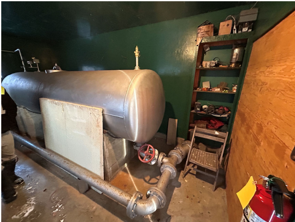
PHOTO 4 – View of pressure tank in Well #1 well house.
