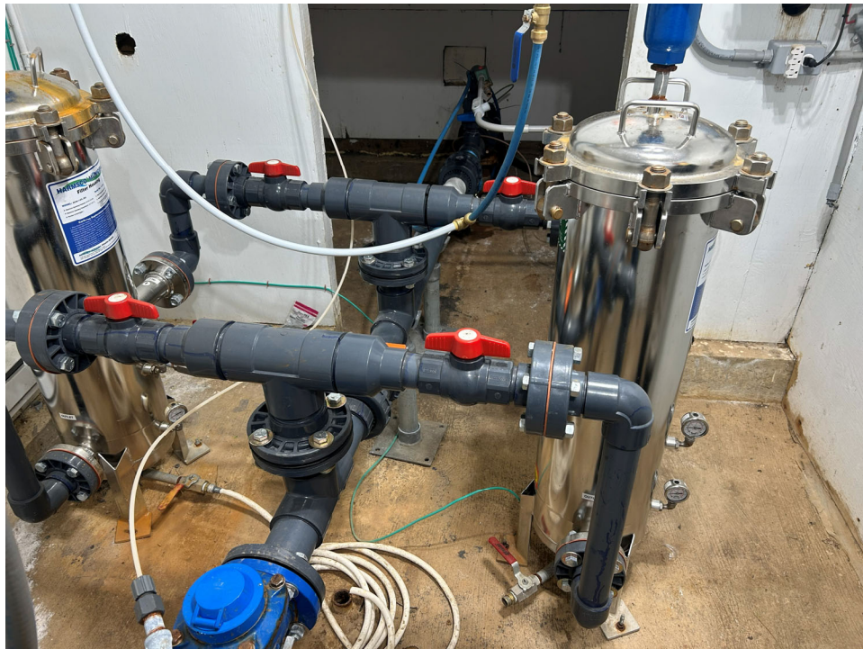
PHOTO 8 – View of filters for Well #2.
